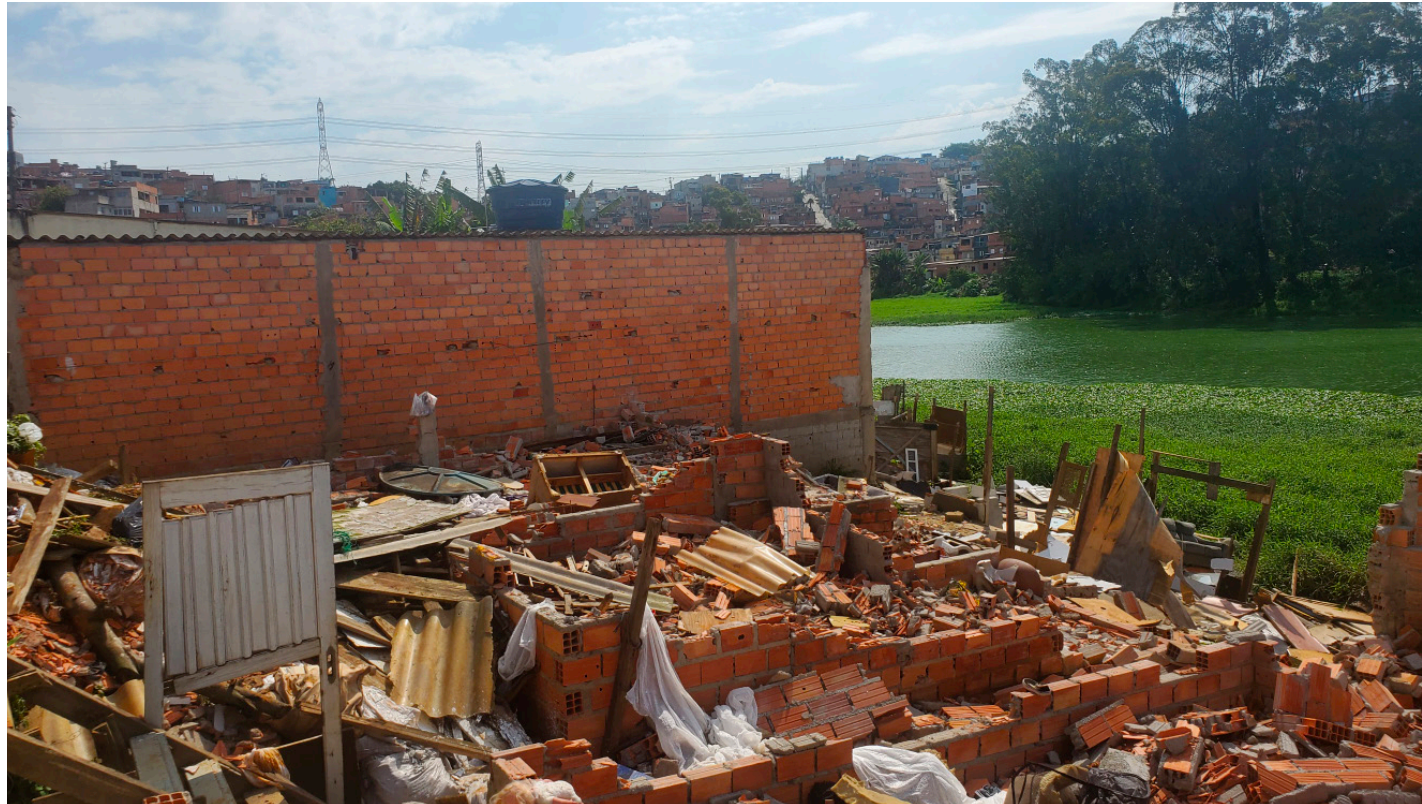
Demolished home of an evicted family in Cantinho do Céu, São Paulo (Author, 2022)
