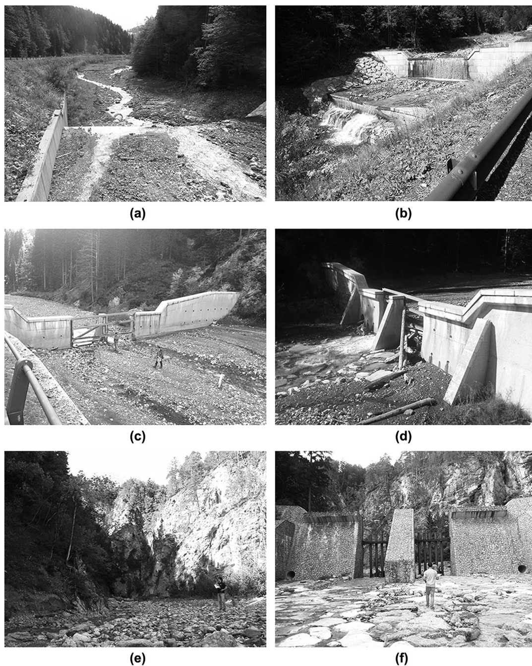
Figure 3. Photos of the structures inspected: (a) downstream view of check dam 1; (b) check dam 1 and sill structures located in series; (c) downstream view of check dam 2; (d) level of obstruction in check dam 2; (e) upstream deposit in check dam 3; and (f) level of obstruction in check dam 3.
