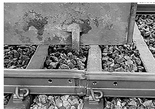
Figure 1-11 Breakage of the rail
