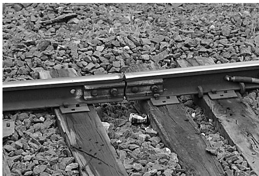
Figure 1-10 Breakage of the Joint bar
