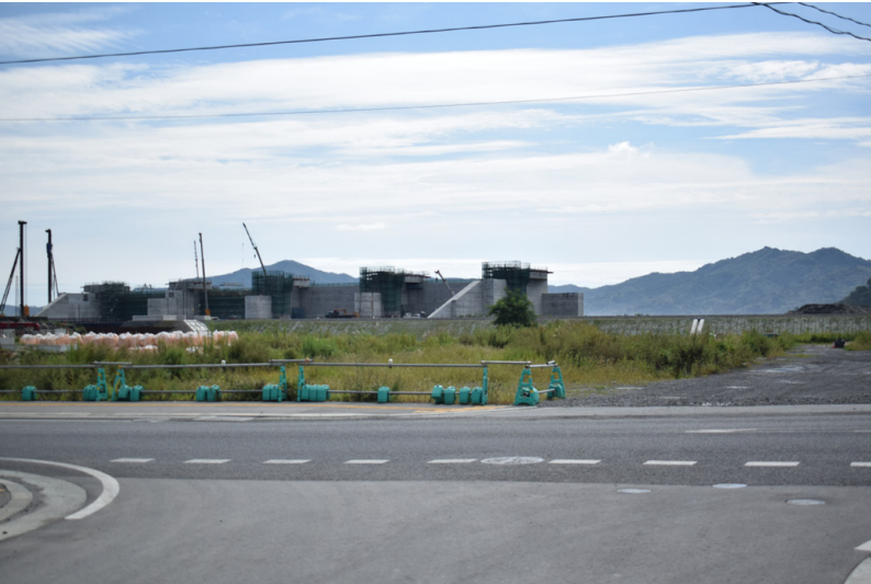
Picture No.80 The storm gate barrier under construction as of 2018 , 7 years after the tsunami. (Author, 2018)
