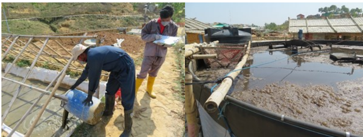
Figure 1-3. Lime treatment of the British Red Cross (left, Rohingya volunteers), aerobic treatment of the International Federation of the Red Cross and Red Crescent Societies (right). Kutupalong camp at Cox's Bazar, Bangladesh, March 2019 (Photo: C.M. Hooijmans)
