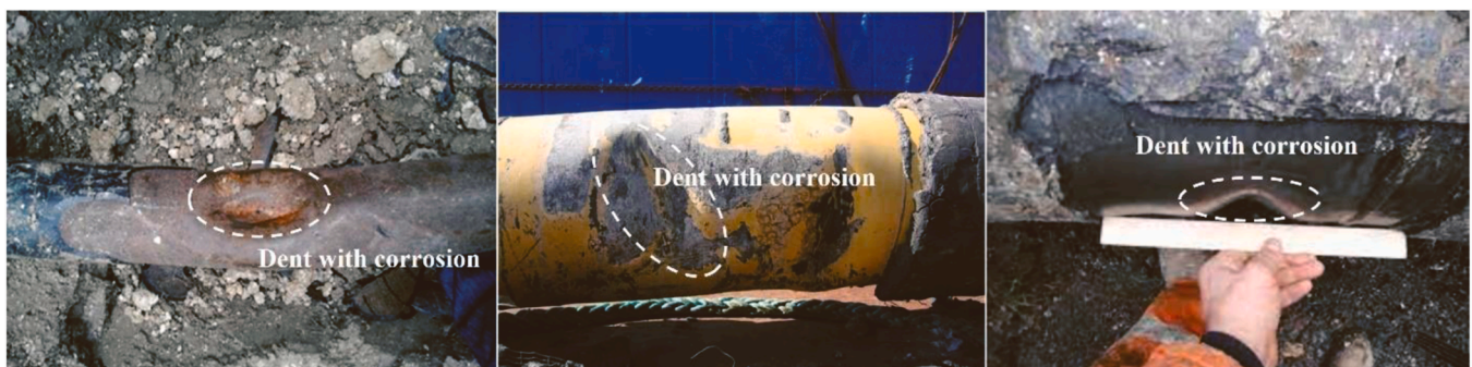
Fig. 2. Dented pipe segment examples with corrosion (Huang et al., 2022a).
