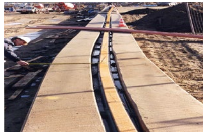
Figure 19. Deformed crane beam due too heavy densification of reclaimed sandfill.
