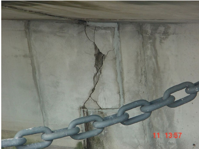
Figure 14. Cracking of concrete structure due to wrong connection.
