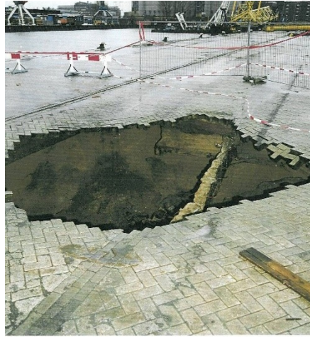
Figure 6. Hole in front wall of caisson quay wall.
