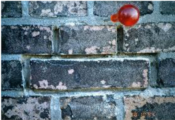
Fig. 18 Weak, decayed trass lime re-pointing
