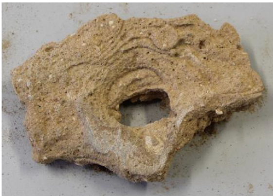
Fig. 28 Deep circular erosion on a render sample of Valflores Palace
