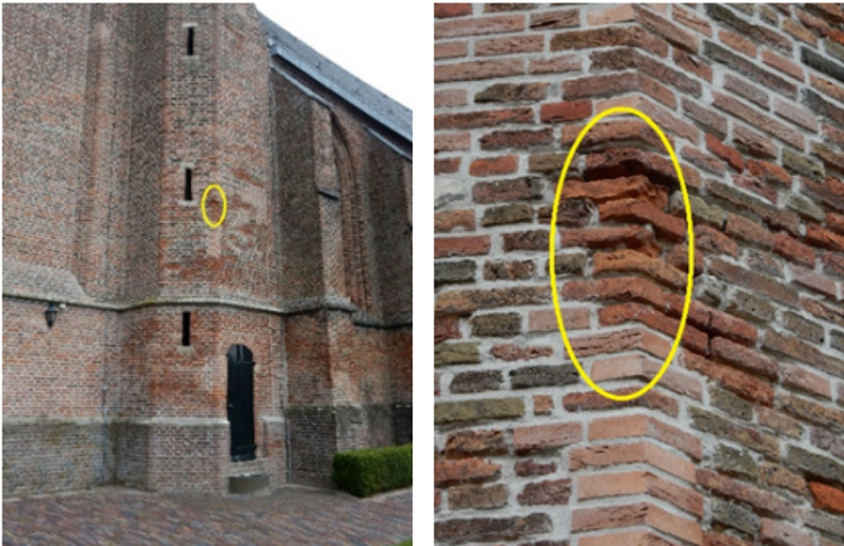
Fig. 21 Situation of the damage in 2016. Left, the reddish parts of the masonry indicate where the repointing is damaged. Right, detail of one of the spots with damaged repointing
