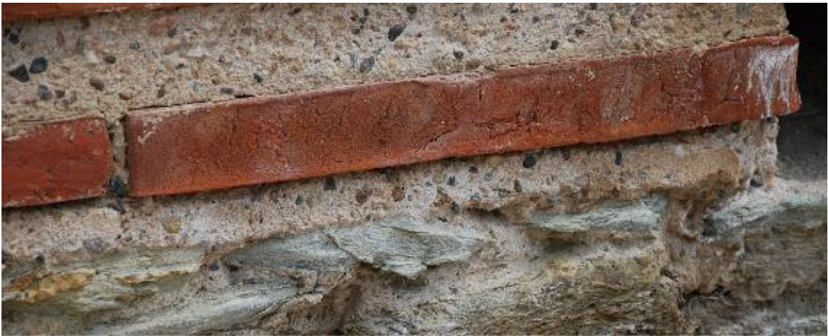
Fig. 30 Repair mortar in a mix structural system of Galerius Palace in Thessaloniki, Greece
