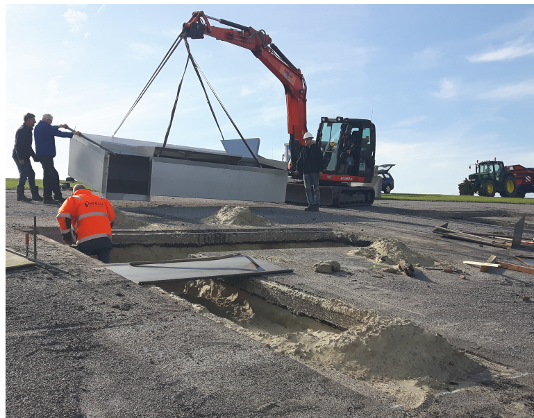
Figure 3: Excavation of the dike slope and placement of the overtopping tanks inside the dike.
