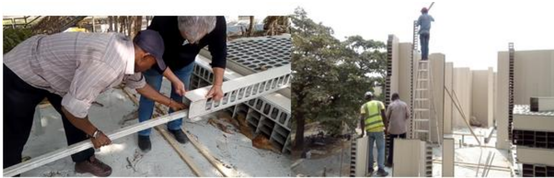
Figure 3. Service duct being inserted on site as worker on the right hammers box and barrel into each other
