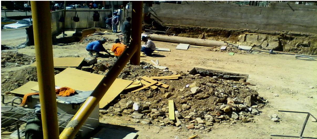
Figure 1. Illustration of poor use of PPEs in Lesotho construction (Source: Authors)
