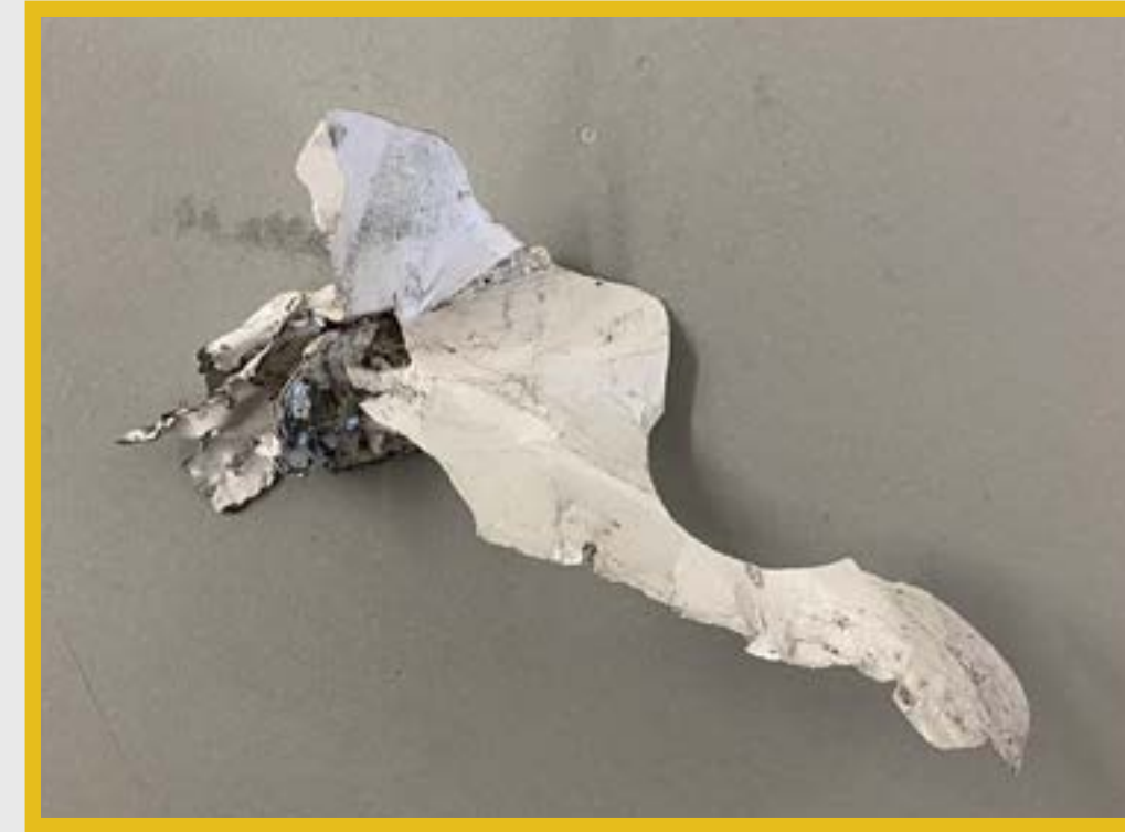
Figure 36. Reflector still stuck to the steel backplate in the CoreLine.
