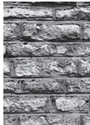
The softness of limestone - decay due to local climate and pollution
