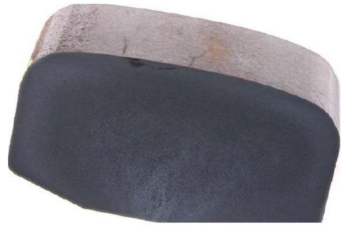
Figure 2. Picture of the examined damaged of the HSL-Zuid. The cracks do not grow into the rail but stay relatively close to the surface (Schalk, 2016).
