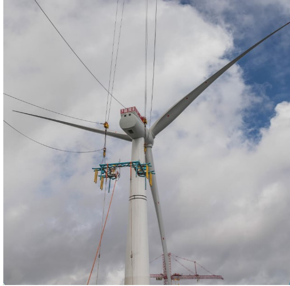
Figure 5.4: The stability frame (blue) as used for the Hywind project by Saipem (SAIPEM, 2017).
