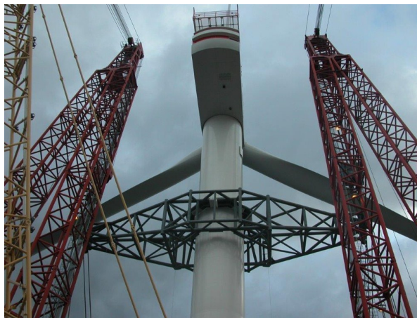
Figure 5.5: The support frame used to hold the wind turbine during installation of the Beatrice project (Scaldis, 2007).
