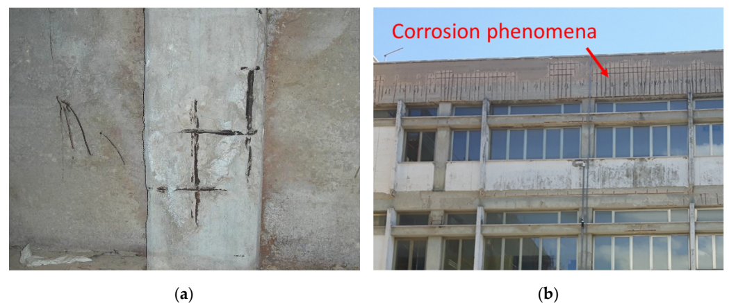
Figure 6. Example of corrosion phenomena to a column in the basement (a) and façade structural members (b) observed during in situ surveys (from UEFA/ELENA research project [23]).
