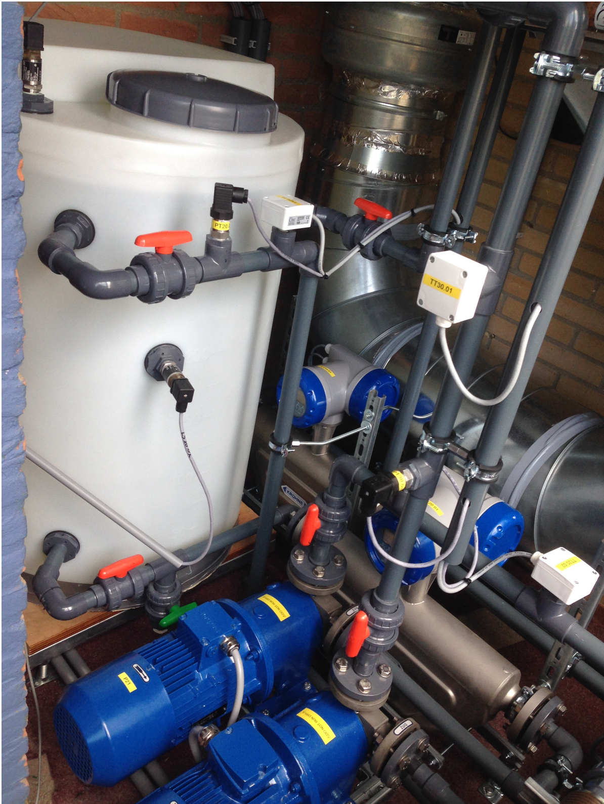
Figure 5.2: A segment of the pilot system in Twello before the application of the insulation material. At the left, the white storage vessel is visible which contains the majority of TBAB solution/slurry. Also, the red valves and the steel air duct in the background are visible. The black sensor heads measure the pressure and are not placed at equal level.
