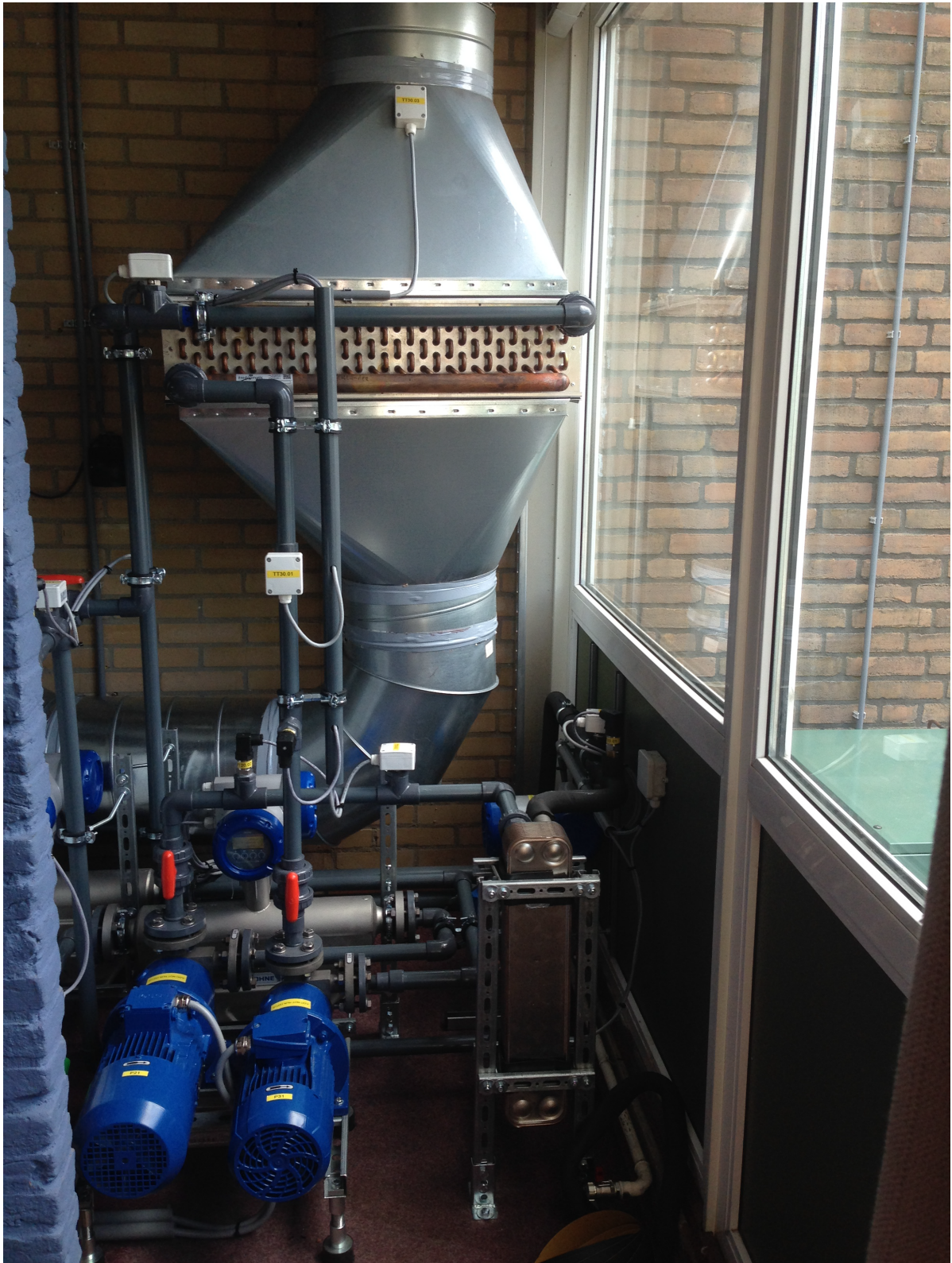
Figure 5.1: A segment of the pilot system in Twello before the application of the insulation material. The air cooler is visible in the top with two exposed headers and exposed bends. Two blue peripheral pumps are placed on the ground. The generator stands next to the pumps. Grey tubes connect the various components to each other. Also, the sensors with yellow labels are visible. The sensors are mainly placed in the middle of the connecting pipes.
