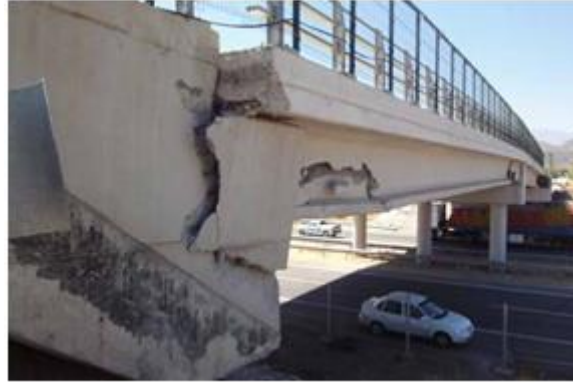
Figure 1.3 Example of a brittle shear failure (Chada Overpass, Chile). [11]
