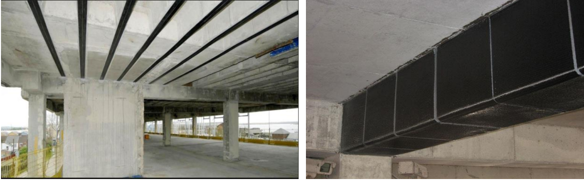
Figure 2.5 Bending strengthening of RC beams using CFRP lamellas (left) and shear strengthening of RC beams (right) using U-shaped CFRP jackets [22] [23].
