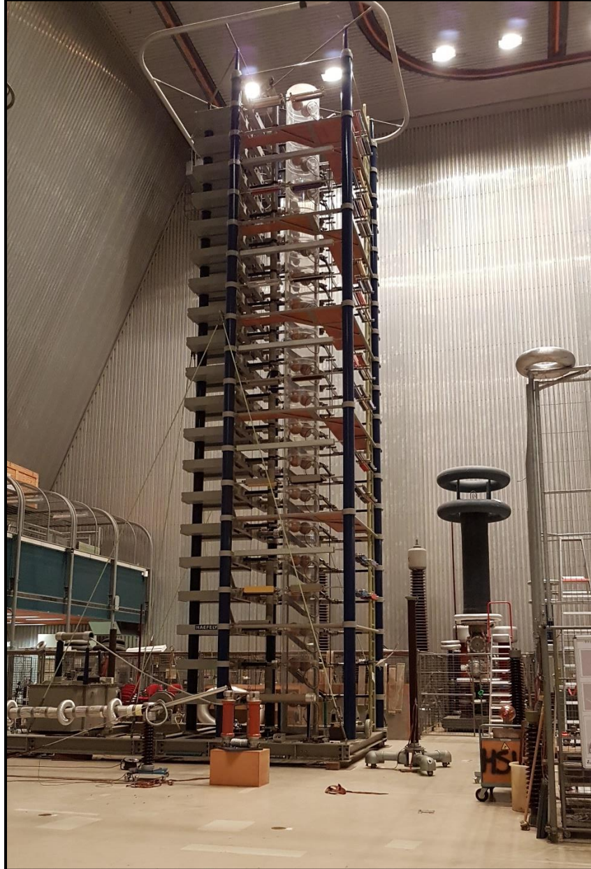
Fig. 5.2: Test setup for Lightning Impulse testing
