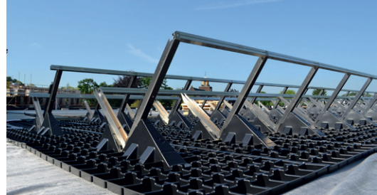
■ Solar roof system from Optigrun (images: Optigrun)
