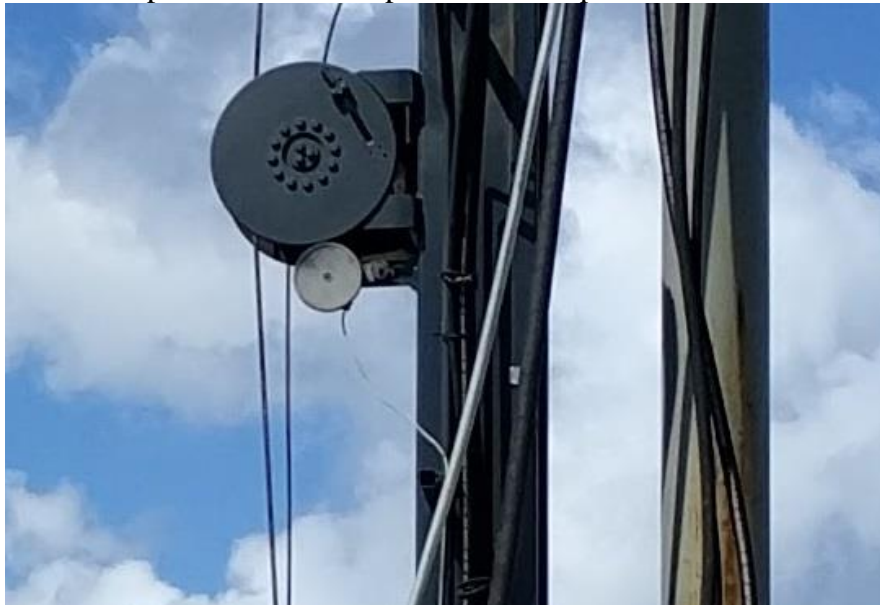
Figure 61: Depth sensor attached to the winch wheel
