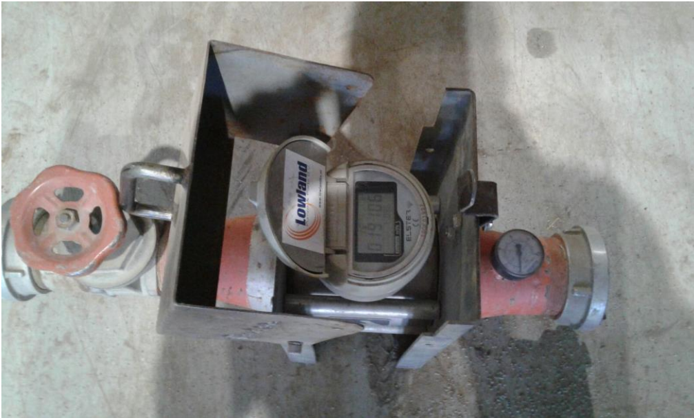
Figure 62: Water pressure and flow sensor
