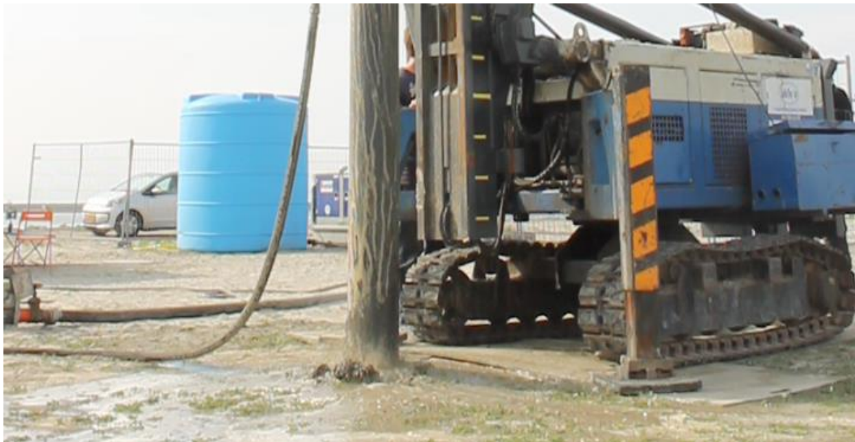
Figure 13: Upwards flow of water forming a lubrication layer between pile shaft and surrounding soil.
