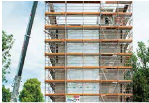
FIG. 9 Facade installation process for the Holz8 building in Bad Aibling (source: www.huber-sohn.de)
