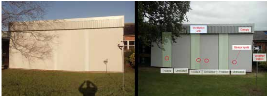
FIG. 6 Demonstrator on a real house façade in Shrewsbury (UK) for outdoor testing
