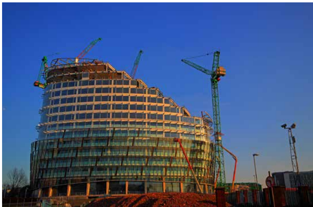
FIG. 2 Construction of the double skin façade at One Angel Square, Manchester, UK (source: Alastair Wallace / Shutterstock.com)
