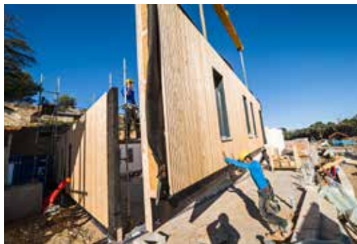
FIG. 11 Facade installation process for the Nexity Ywood «L'Ensoleillée II» building in Aix-en-Provence (source: © Nexity, Yann Bouvier)
