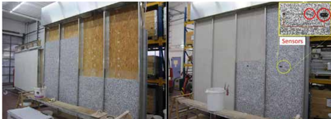
FIG. 4 Construction of the demonstrator wall consisting of ETICS, sensors and ventilation unit
