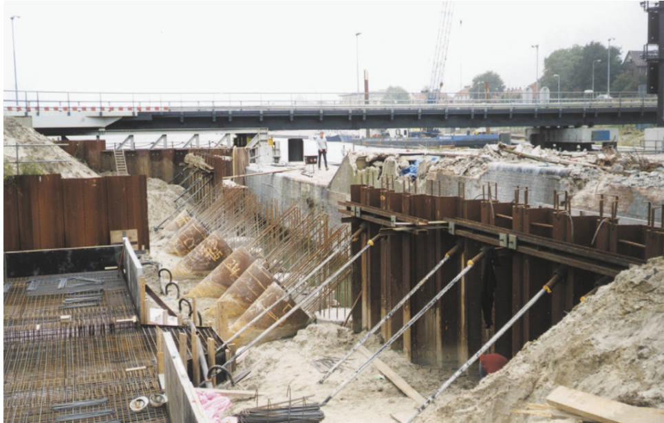
Figure F.5: Strengthening of lock head of the Southern lock in IJmuiden. Retrieved from (Beem et al., 2000).
