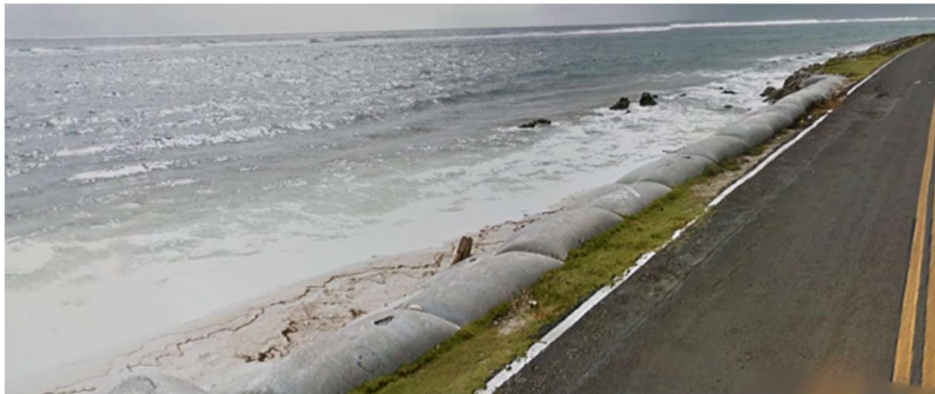
Figure 1.2: Placement of sandbags in order to protect the road along the southeast coast of San Andrés against coastal erosion (Klooster, 2020).
