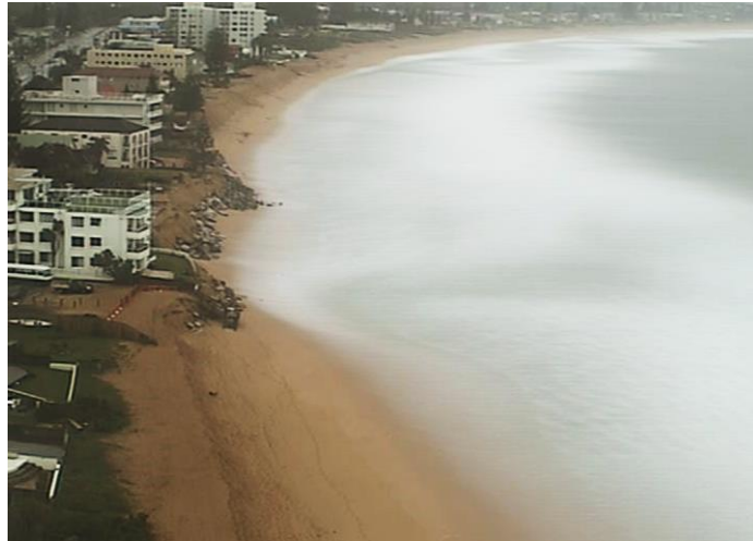
Figure 2: Further coastline erosion will endanger the stability of the buildings (Davidson et al., 2013)
