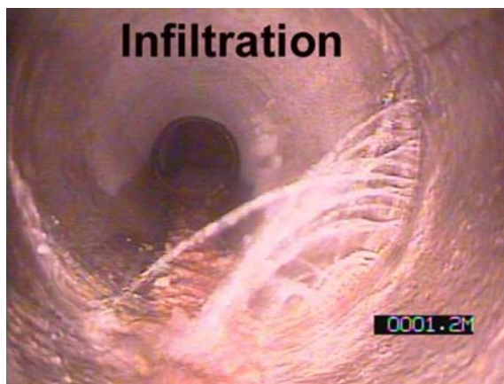
Figure 3.47 Clear example of infiltration of groundwater into a sewer pipe. Source: Deltares.
