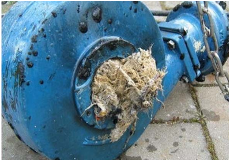
Figure 3.43 The cause of an increase in energy consumption became immediately clear when inspecting the pump. Source: courtesy Kees Kooij (Deltares).
