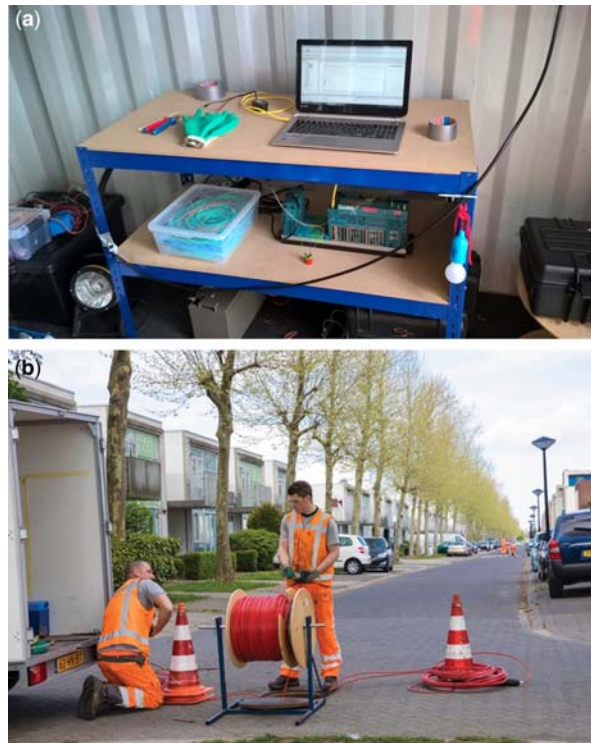
Figure 3.51 (a) DTS measuring computer, (b) Installation of a DTS cable. Source: courtesy Rémy Schilperoord (Partners4UrbanWater).
