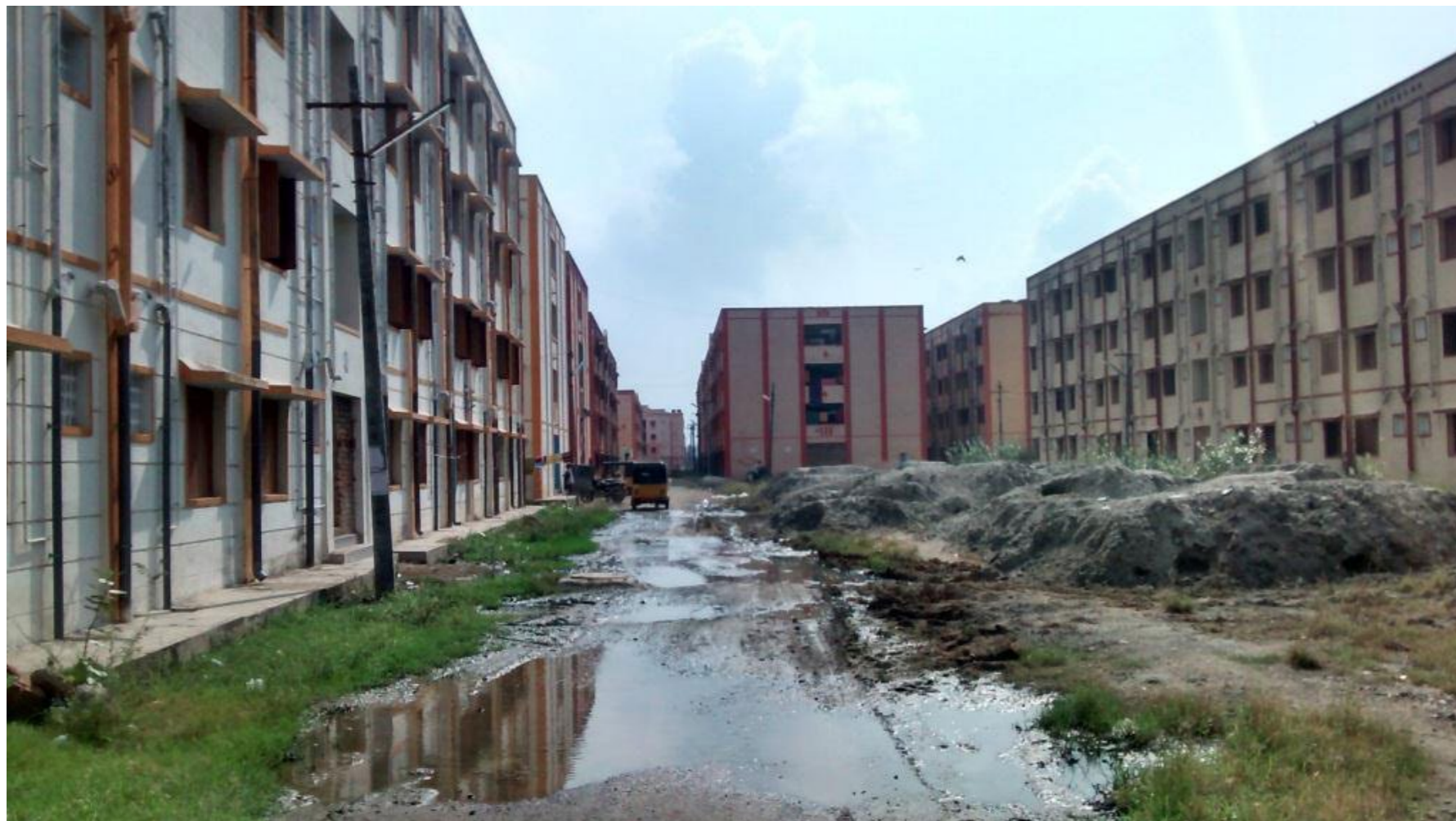
Source: TNSCB resettlement tenements at Ezhil Nagar seen flooded with sewerage water: a sorry state of affairs.
