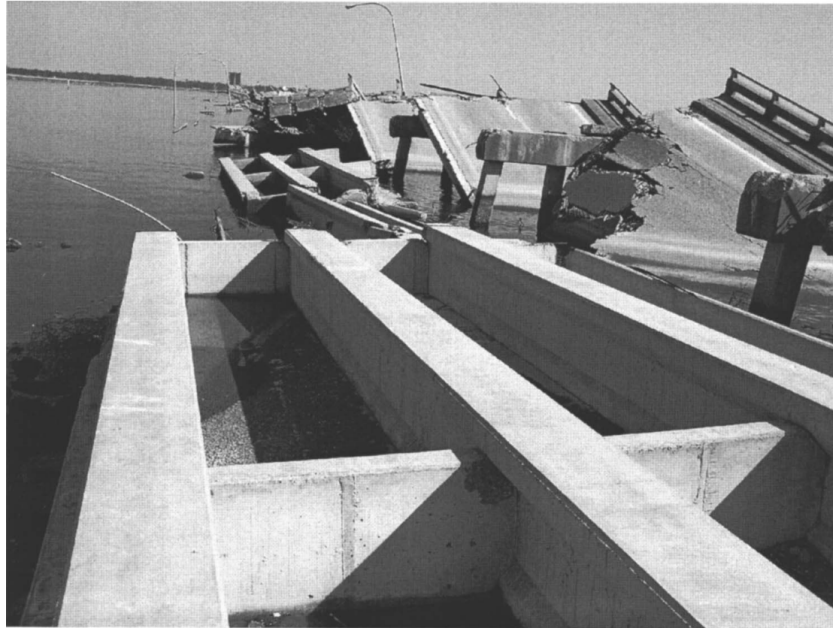
Figure 1.1: Damage on bridge decks caused by wave impacts during hurricane Katrina (Robertson et al. (2007)).
