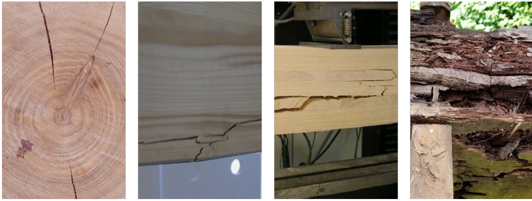
Figure 2.7: Types of failure (F.L.T.R.); cracks (Wikimedia Commons, 2005), bending failure (Franke et al., 2015), shear failure (Schmid et al., 2010) and insects and fungi (Wikimedia Commons, 2020)
