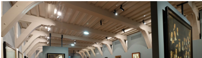
Figure 7.1: Monumental timber floor ceiling of the dormitory in the Prinsenhof Museum in Delft [Figure from ABT]
