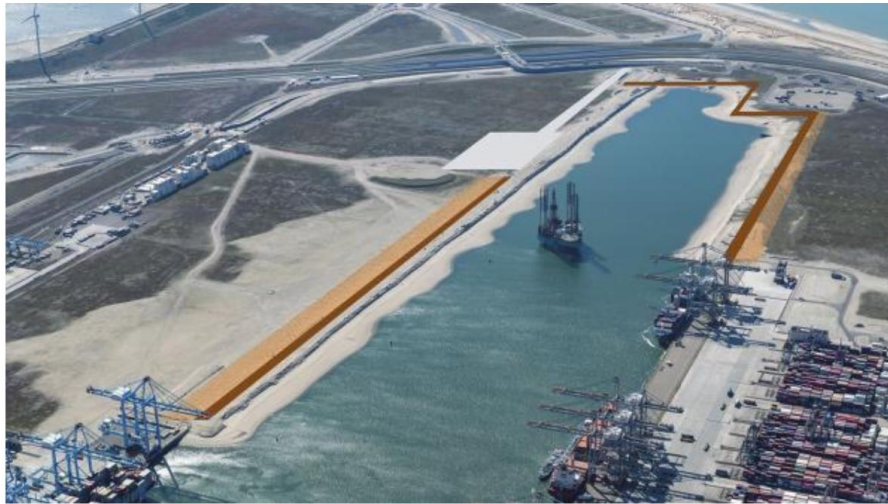
Figure 1.1-2: Expansion of Prinses Amaliahaven's quay walls (Port of Rotterdam website: Ongoing Projects: Quay Wall Construction Amaliahaven).
