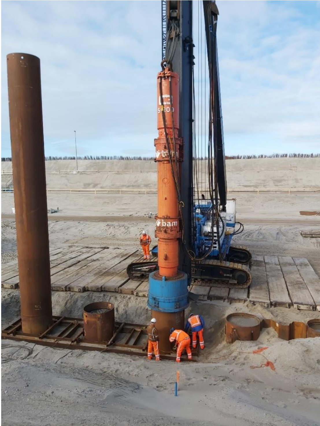
Figure 5.2-3: Installation of steel open-ended combi-wall pile with the IHC-S 200 hydraulic hammer (photo personally taken).
