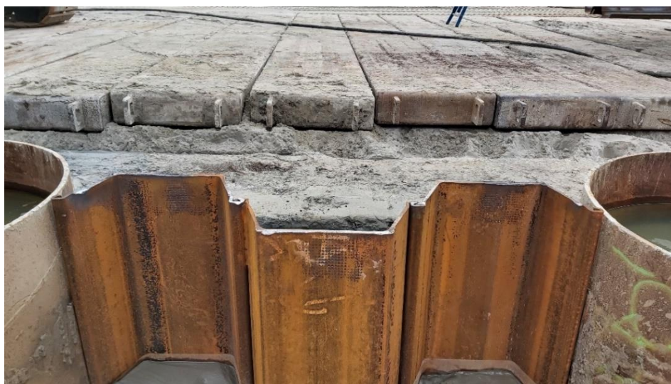
Figure A 5: Combi-wall piles and sheet-pile wall installed to final depth (photo personally taken).
