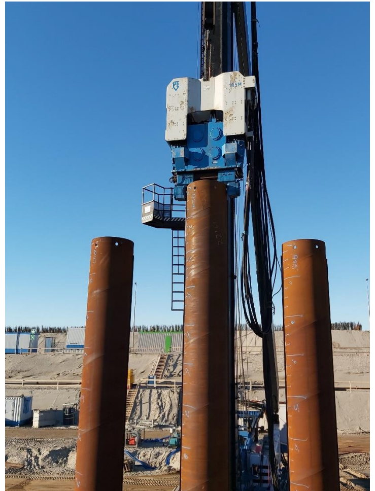
Figure A 2: Partial installation of combi-wall piles with the vibratory hammer (photo personally taken).
