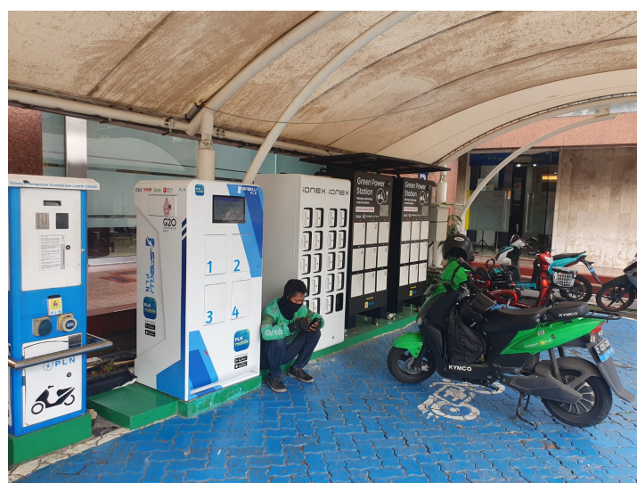
Figure 4.9: Multiple Battery Racks from Different Providers in One Place
