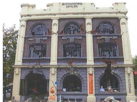
Figure 2.15 Failure of spandrels resulting in slender piers [21]
