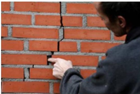
Figure 1.1 Typical crack in the URM wall
