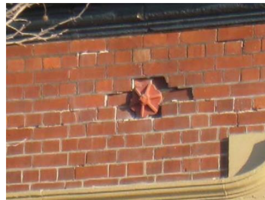
Figure 2.18 Punching shear failure of wall at anchor plate [23]
