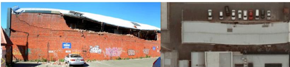
Figure 2.16 Out-of-plane wall failure due to excessive roof diaphragm displacement [22]
