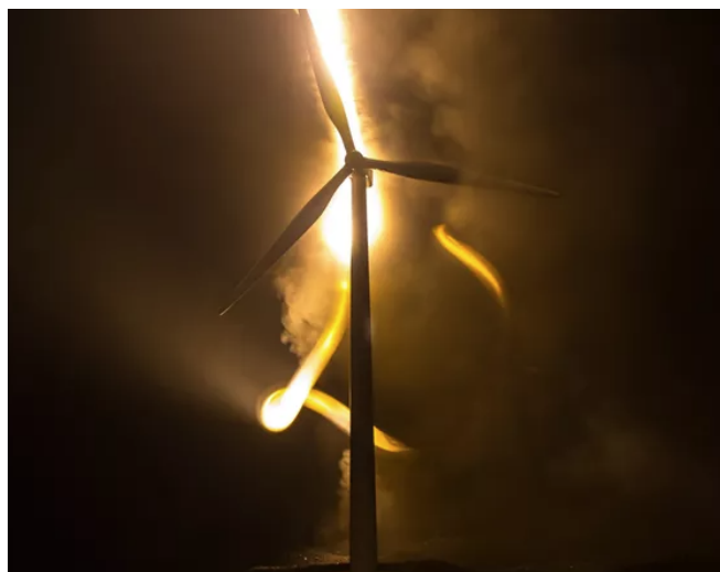
Figure 1.2: Wind turbine catches fire due to lightning strike (Senn, 2022)
