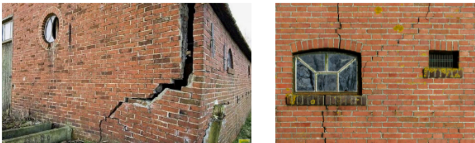
Figure 1.1: Damage to unreinforced masonry structures due to earthquakes.
