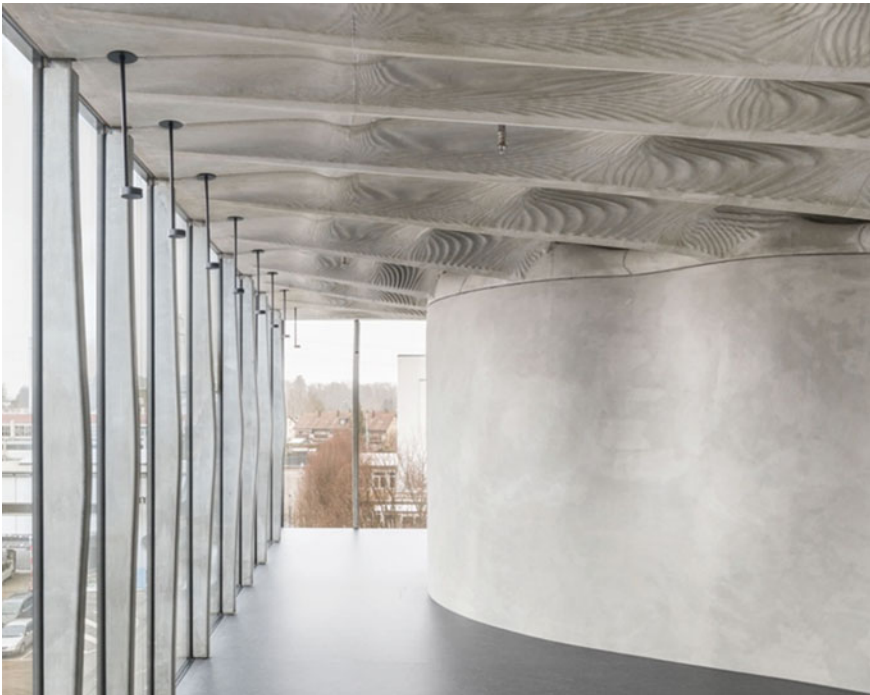
Fig. 2.16 Final installation of façade mullions in the DFAB House, on the left-hand side of the image
