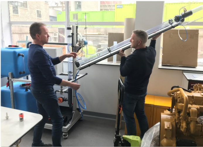
Fig. 1: Installation of the fluidisation expansion column at the QMUL Engineering Building in London.
