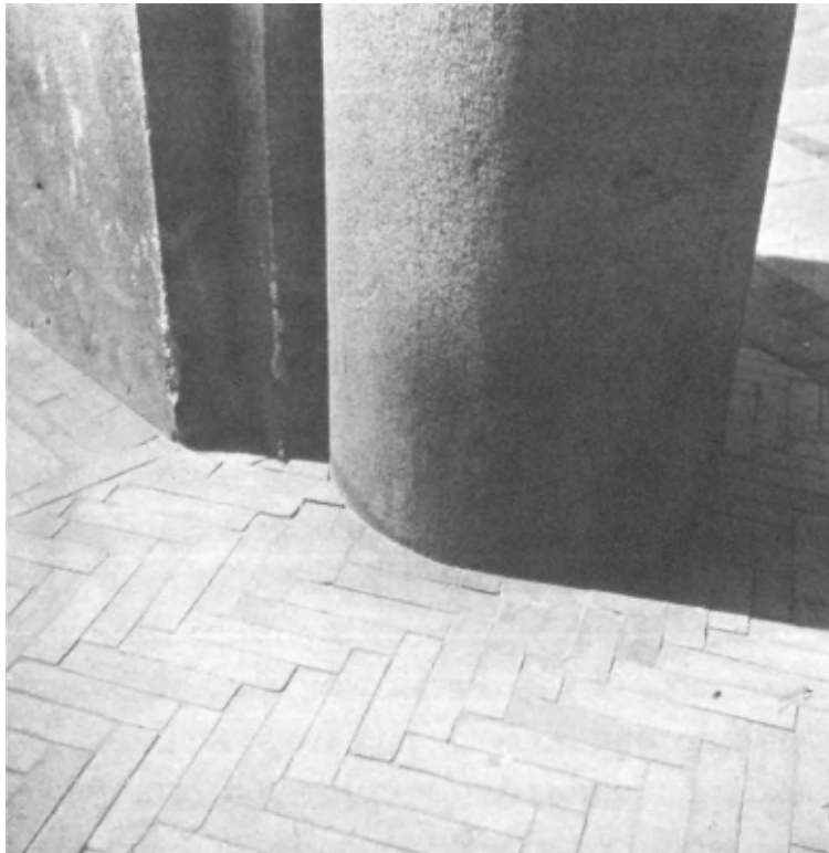
Heavy granite column stands directly on lighter paving shattering it. Collonade in Copenhagen.
