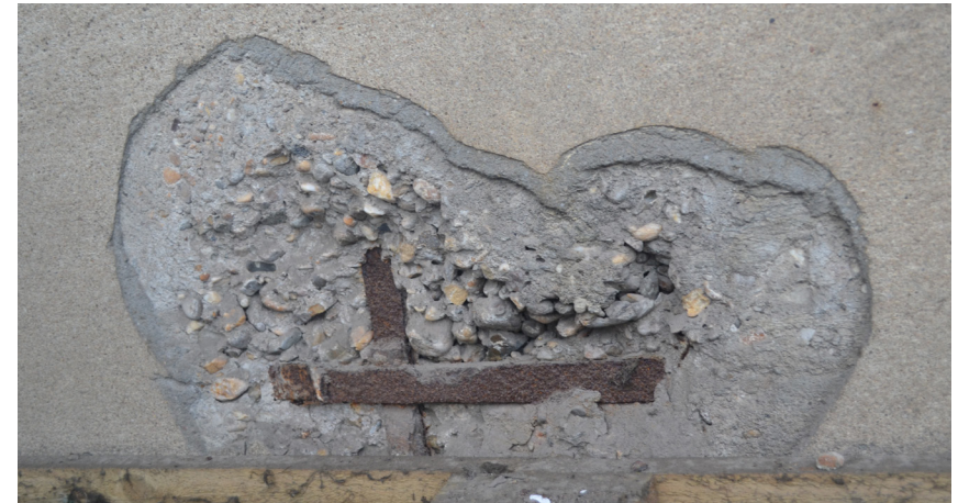
Damaged part of the facade. The different layers are clearly visible: steel reinforcements, concrete with a high amount of aggregates and two layers of surface finish, own photo (2016).
