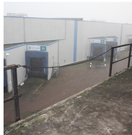
Railing with inexplicable openings, own photo
