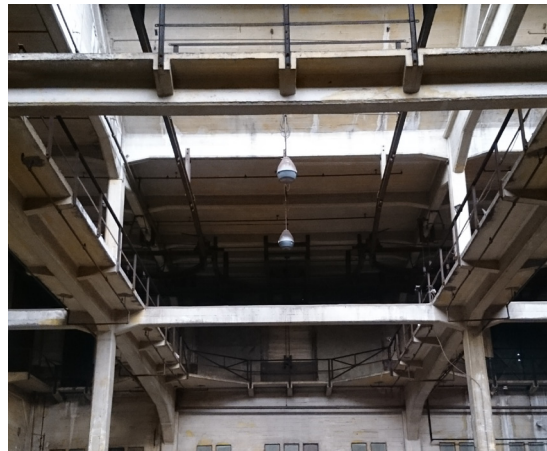
The walkways on the first floor are valued highly. They show how the building used to function, own photo (2016)
