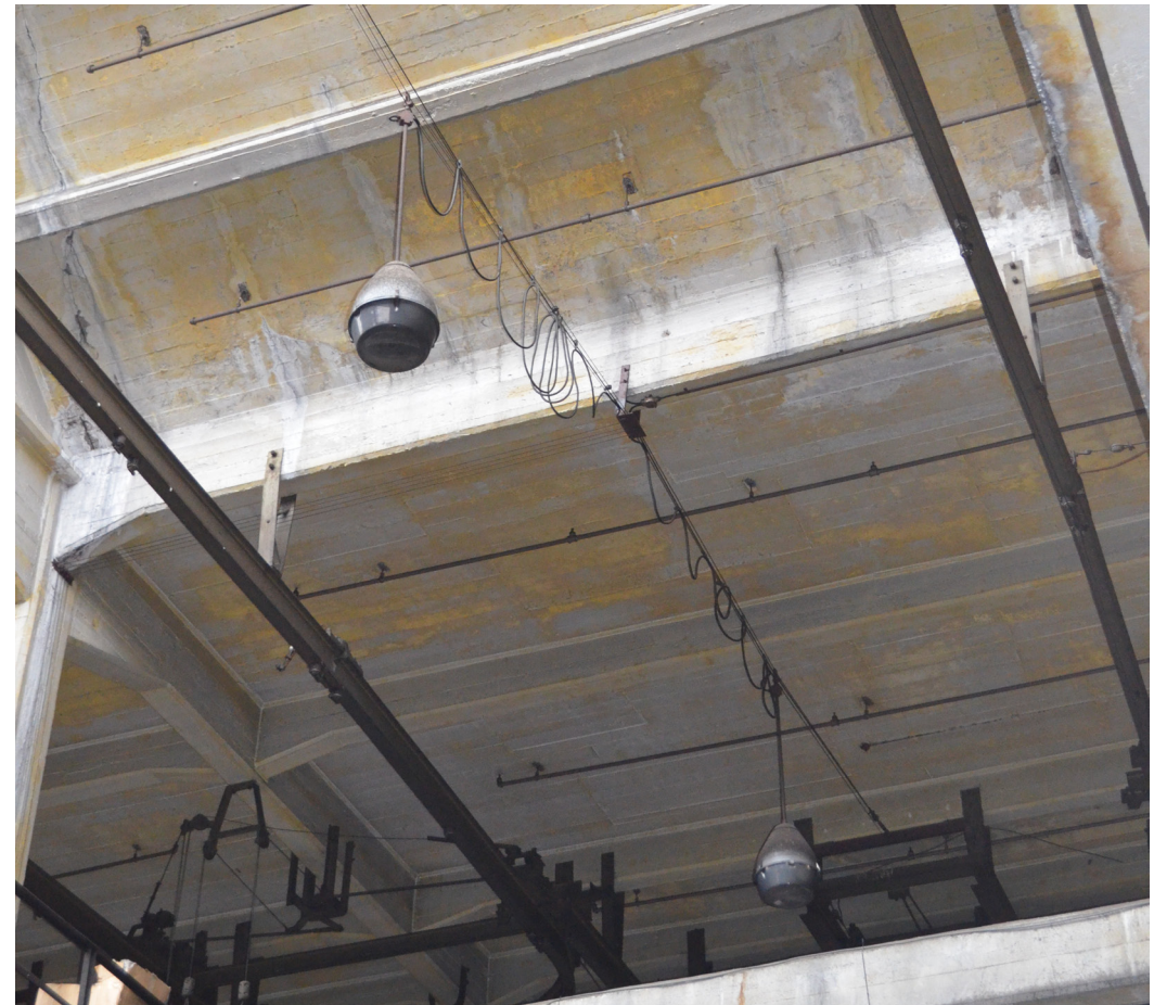
Lighting fixtures in the Katoenveem could be moved, own photos (2016).
