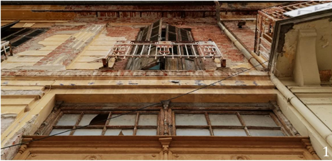
Deteriorated Facade_ Bottom view (Survey Product)
