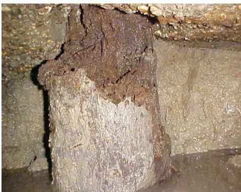
Figure 6.1: Degradation of timber pile [56]
