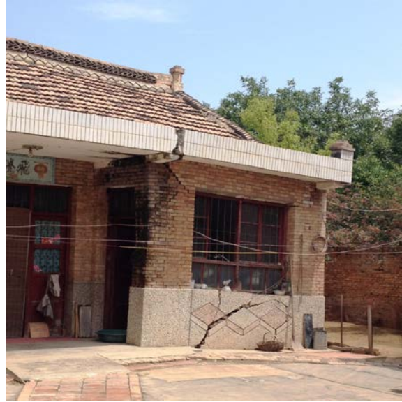
Figure 21 A damaged house in Caizi village, Peixian
