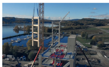
The glulam was erected in large pieces, which were assembled together onsite (Abrahamsen, 2018)
