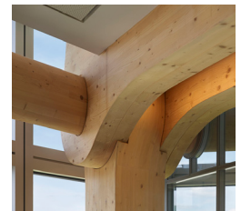
Close up of the structural detail in the finished building ("Tamedia Office Building / Shigeru Ban Architects," 2014)
