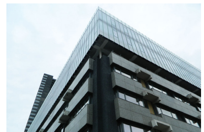
Close up of the detail of the steel columns on top of the renovated building (Pieters Bouwtechniek, 2019)
