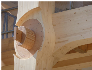
Picture of the spruce pine column to beam connection, using a large LVL dowel of beech for a rigid connection (Hill, 2014)
