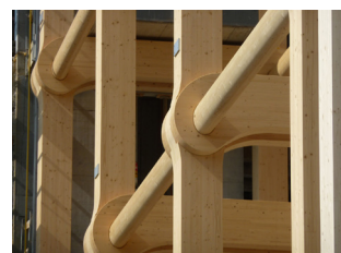
Transverse oval beams connect the portals rigidly to the existing structure ("Tamedia Office Building / Shigeru Ban Architects," 2014)
