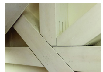
Finished detail of the glulam trusses (Kleppe & Abrahamsen, 2016)
