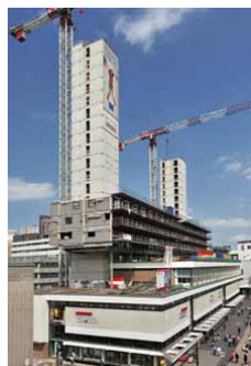
Construction of the extension with the concrete cores and steel structure (Ibelings & van Tilburg, 2013)
