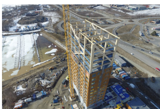
The construction in process showing the large glulam elements forming stable trusses (Abrahamsen, 2018)
