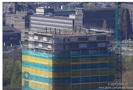
Steel columns are used for the load bearing structure and the outrigger (Skyscrapercity, 2012)
