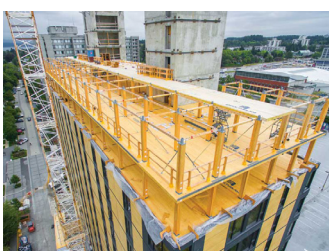
The construction in process, showing the build up of the structure (Metras, Austin, & Fraser, 2016)
