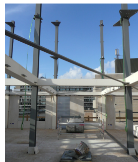
Close up of the steel column and beam structure of the extension (Nationale Staalprijs, 2012)
