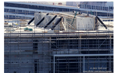
Connection of the steel diagonals of the outrigger with the concrete core (Skyscrapercity, 2012)
