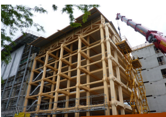
The construction in process, the building was erected bay by bay ("Tamedia Office Building / Shigeru Ban Architects," 2014)
