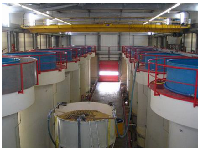
Fig. 1. Full-scale pellet softening reactors located at Waternet (Amsterdam, the Netherlands). The unit consists of 12 Amsterdam reactors with reactor diameter D = 3.0 m (van der Veen and Graveland, 1988).
