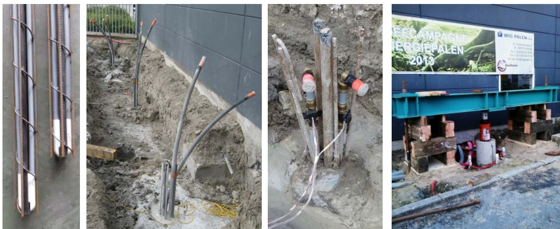
Figure 18: Energy piles installed for a BBRI test program in Ostend (Belgium). The heat exchangers are attached to the reinforcement cage prior to installation. The energy piles are fully monitored with strain and temperature sensors.
