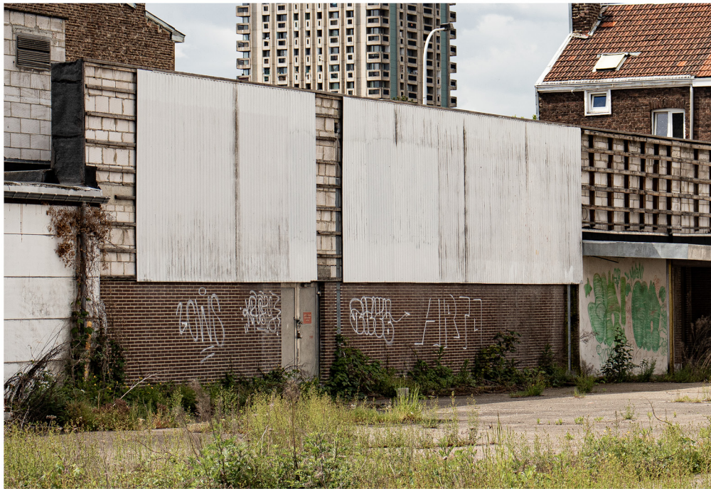
corrugated sheeting, brick work, door, timber framing, concrete masonry (picture by author)
