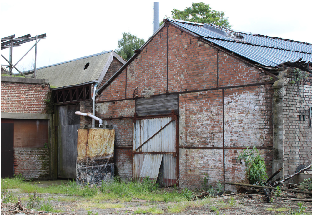
brick masonry, corrugated sheeting, sliding door, straight truss (picture by Wiktoria Paszek)
