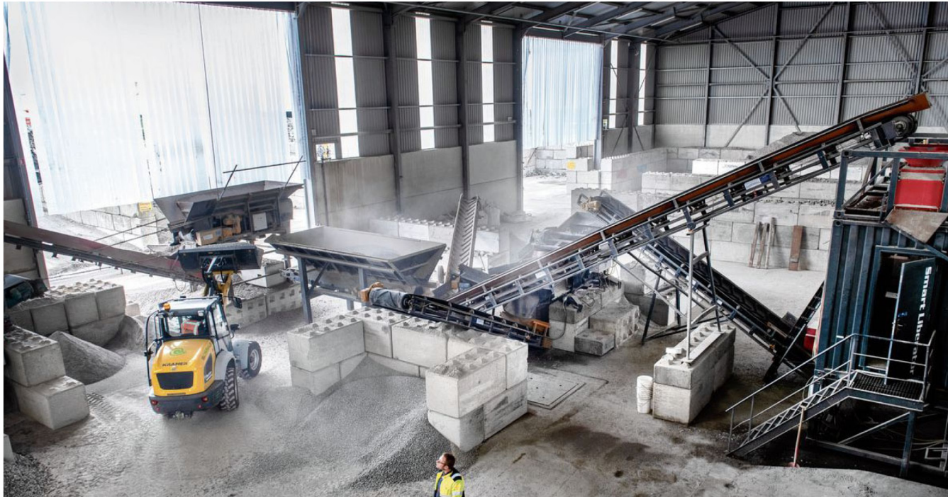
the smart liberator concrete recycling facility, Zaandam, © New Horizon
