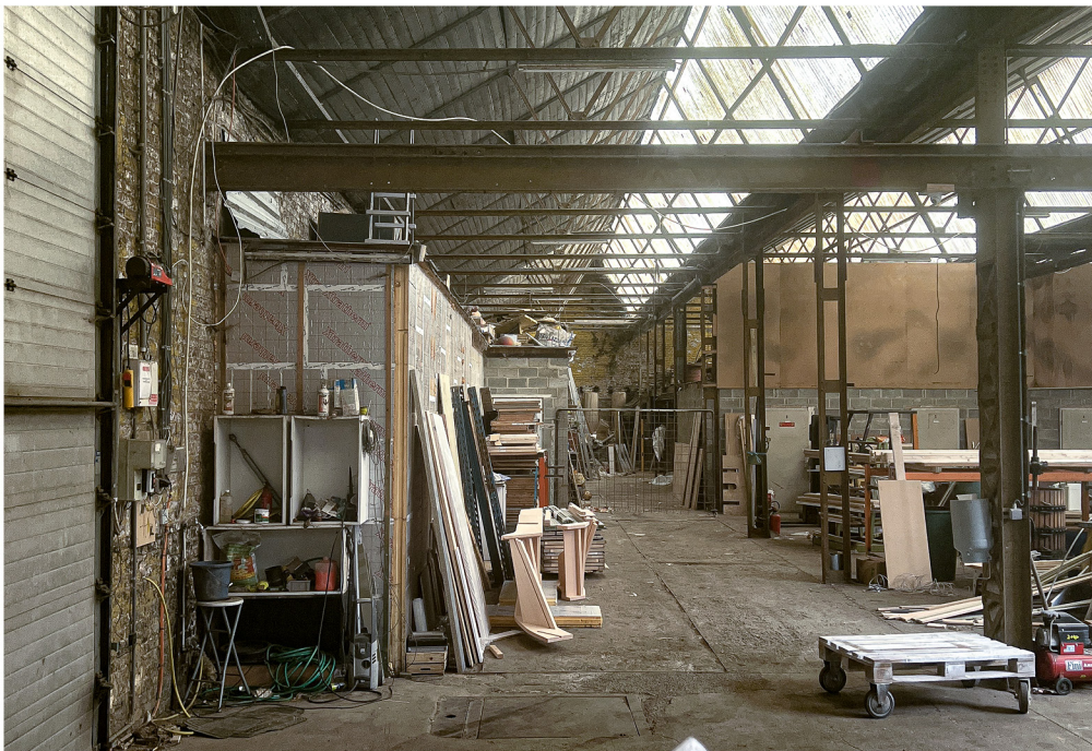
brick masonry, roller door, belgian truss, column, roof decking (picture by Simon van Soolingen)
