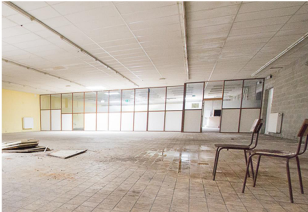
suspended ceiling panel, floor tiles, concrete masonry room divider, radiator, fixture (picture courtesy of realo.be)
