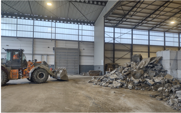
New Horizon urban mining facility Zaandam, © author
