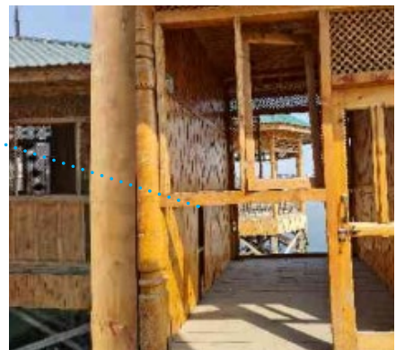
Fig: Vandalized Pavilions newly constructed for the Bab Demb Lake Revitalization Project
