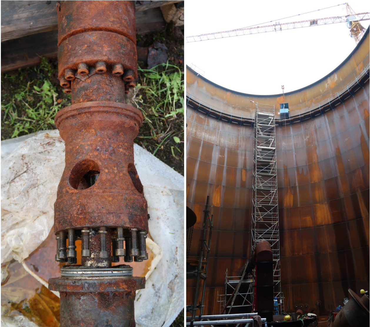
Figure 6: Left: Corroded well pump of the cold well of the HT-ATES in Neubrandenburg. Right: Artificial storage tank to balance short-term supply-demand mismatch.
