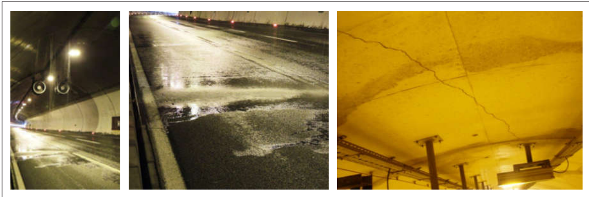
Figure 1 Heavy leaking through tunnel lining and water on the pavement as a consequence influencing traffic safety; cracks on tunnel ceiling [4]
