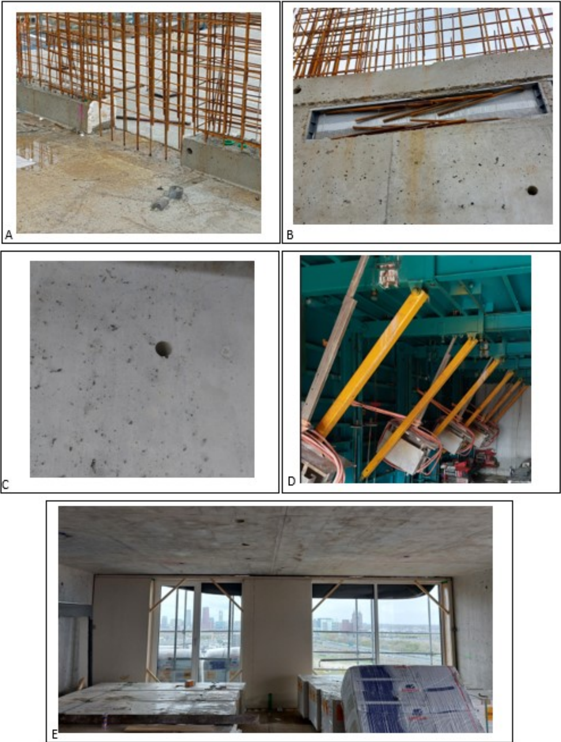
Figure 2.3: Details of the tunnel formwork building method. A: Kickers + starter bars. B: Continuity strip. C: Ties. D: Heaters. E: Precamber.(source: own photo's)
