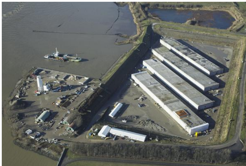
Figure 6.10: Bouwdock Barendrecht during the construction of the tunnel elements of the Tweede Coentunnel
