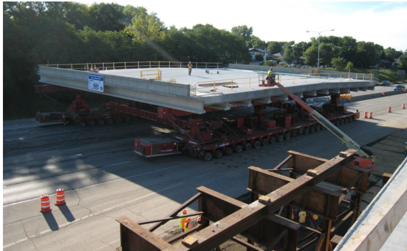
FIGURE 4.13: Superstructure movement by SPMT to the bridge location [Federal Highway Administration, 2015b]
