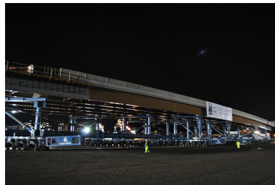
FIGURE 4.15: Superstructure movement by SPMT to the bridge location [Florida International University, ndc]
