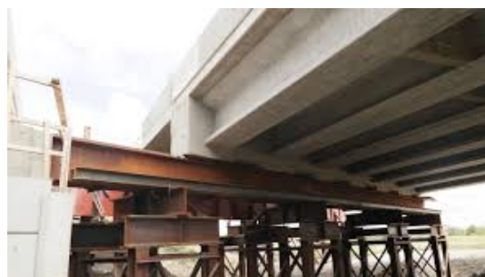
FIGURE 6.6: Lateral sliding of a bridge superstructure [Ohio DOT, nd]
