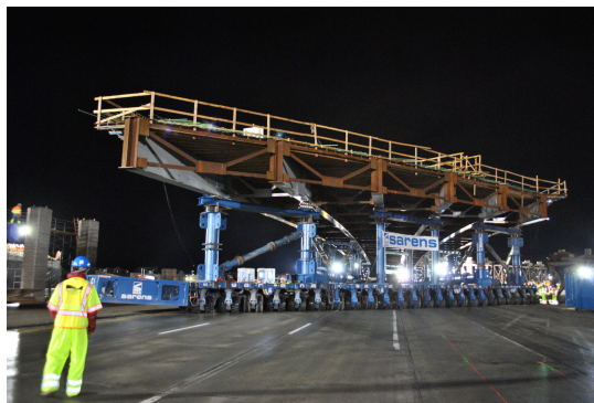
FIGURE 4.14: Superstructure movement by SPMT to the bridge location [Florida International University, ndc]
