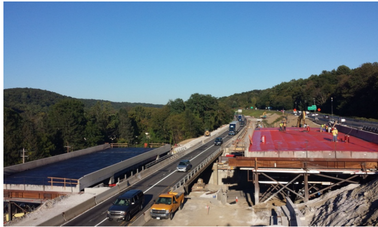
FIGURE 4.7: Construction of two adjacent replacement bridges with differential elevation [Federal Highway Administration, 2014a]
