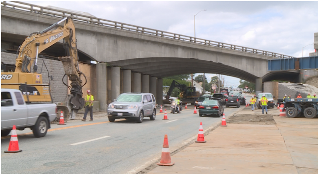
FIGURE 4.21: Construction of the GRS-IBS substructure behind the existing interior supports [Turn To 10, nd]
