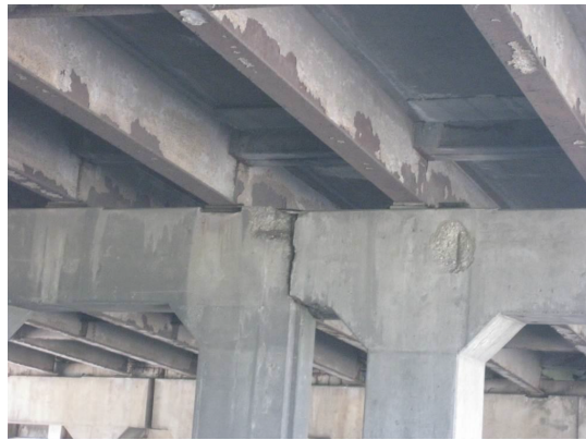
FIGURE 4.11: Poor condition of the concrete pier in the Maryland Avenue Bridge [Federal Highway Administration, 2015b]
