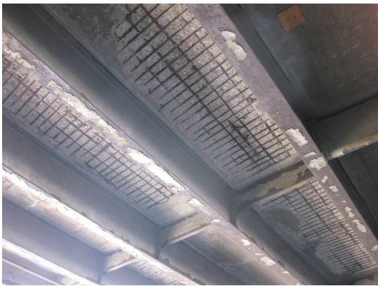
FIGURE 4.10: Poor condition of the concrete cover in the Maryland Avenue Bridge [Federal Highway Administration, 2015b]
